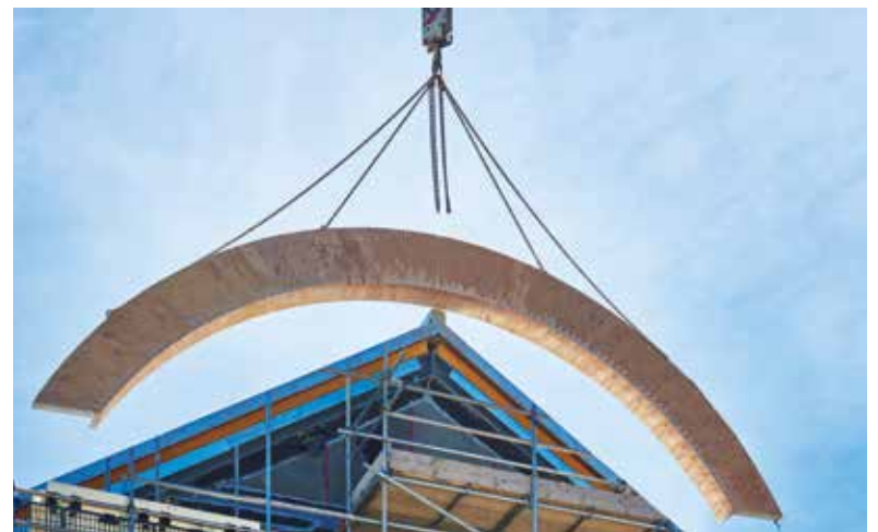
9.6m Stainless Steel Brick Slip Feature Lintel installed at DNRC, 1 of 1,000 lintels supplied.
